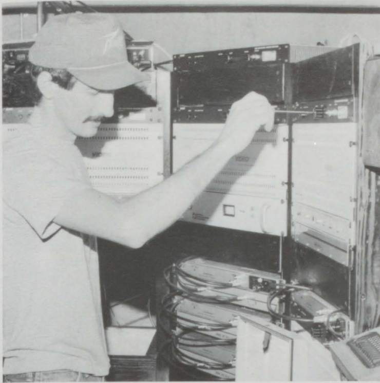
Cable installation was almost completed when the Lion went to press. Above, Paul McCully of Corrine Cable System of Stillwater was snapped checking a junction box to make sure that the signal is going to the proper locations.
